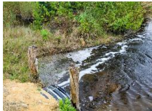
Fig. 8c On the main road crossing FCFR, only one very small culvert (50 cm diameter) connects the two halves of a lagoon system that was split by the construction of the road.
